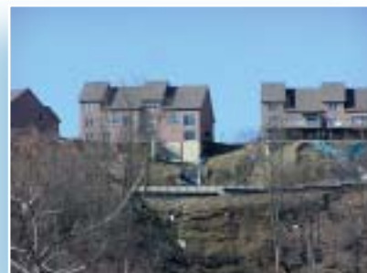
Tree removal and grading too close to the ridgeline caused a serious landslide exposing building foundations. Walls are being built in an attempt to stabilize the site, and black plastic being used to prevent water from further saturating the soils. This landslide scar will take decades to heal.
